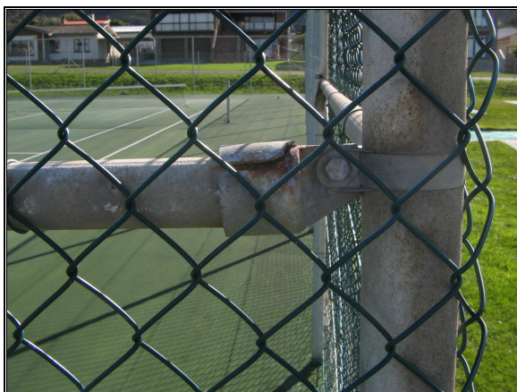
Rail corner connector that needs replacement
